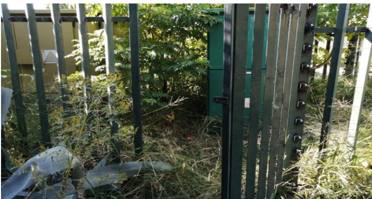
Fig 8: No Padlock on the inside gate of the Eskom Transformer
