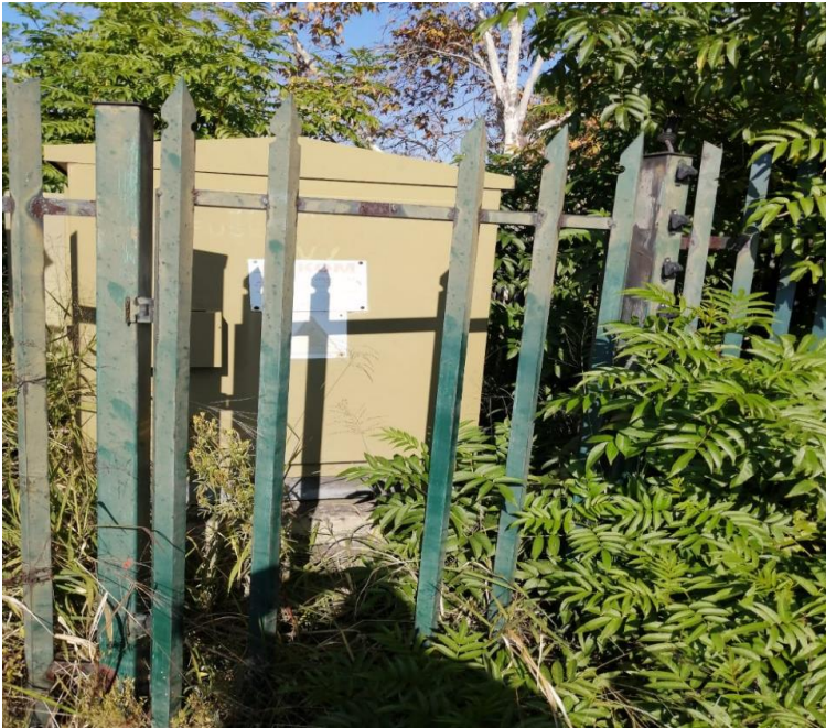
Fig 7: A missing palisade pole of the Eskom transformer providing an entry into Woodrock
