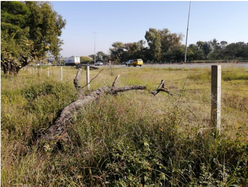
Fig 5: A tree has fallen on the perimeter fence creating an entry/exit point off the highway.
