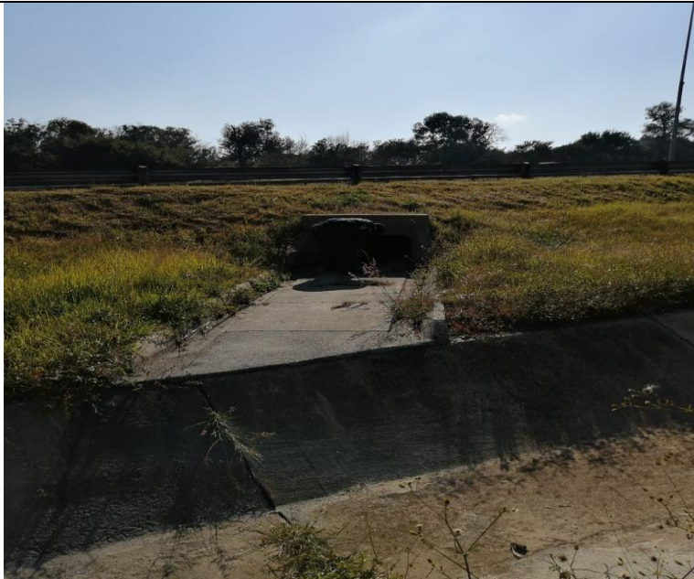
Fig 9: Storm drain tunnel connects Woodrock to the squatter camp across the highway
